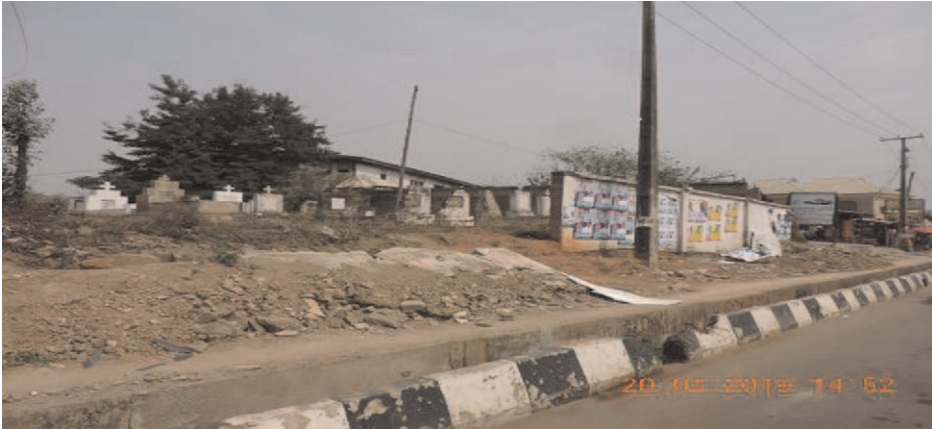
FIGURE 6. The perimeter fence of a cemetery at Iyana Mortuary in ruins after several years of road expansion. Photo by Olasupo Thompson.
